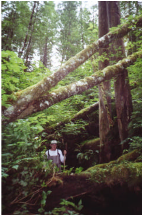
Photo 7. An upstream view of the channel where the railway trestle has collapsed.
