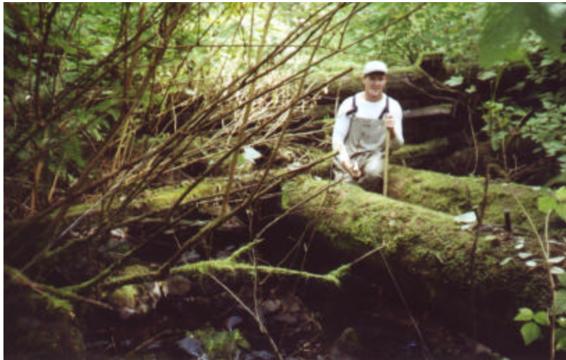
Photo 5. An upstream view at the downstream end of the collapsed trestle. The channel flows underneath the debris.
