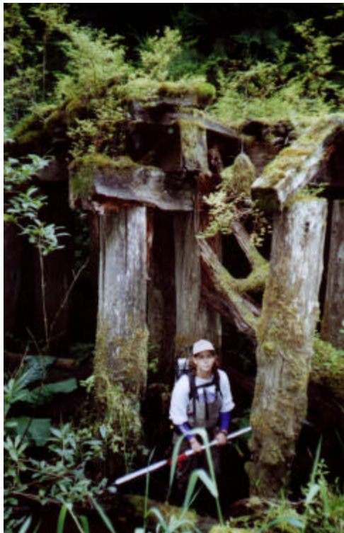
Photo 2. A downstream view of the railway trestle, most of which is still standing in the channel in Site 1.
